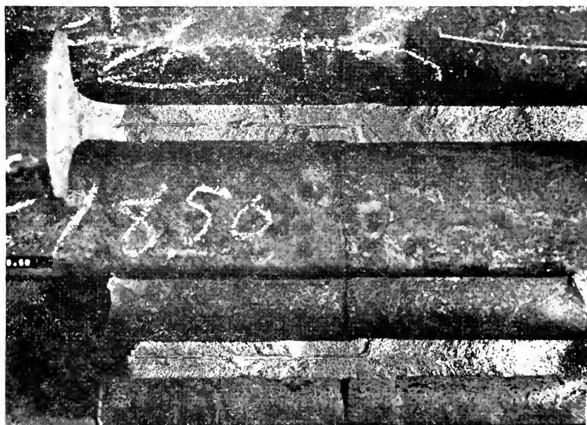
Fig. 10 (Investigation 136-27, Sample B)—Fractured faces of the specimen shown in Fig. 9. The line in the center of the web on the left side of the weld indicates that a pipe is present in the east rail.
